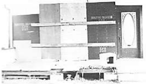
Damage Caused by Automobile
